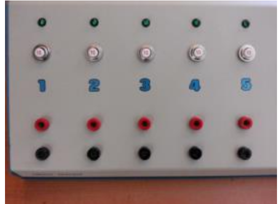
Figure 27 Front panel connections, circuit breaker buttons, and LED indicators.
